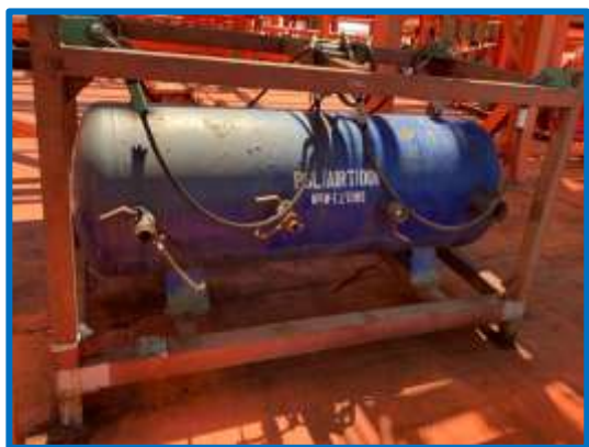
BA Air Accumulator Tank
