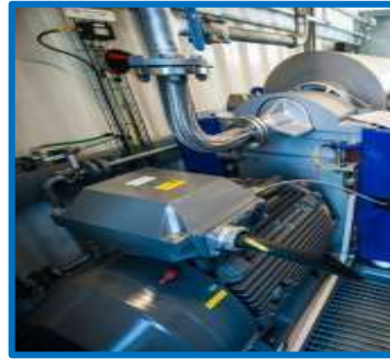
ATC 3-PHASED DECANTER
